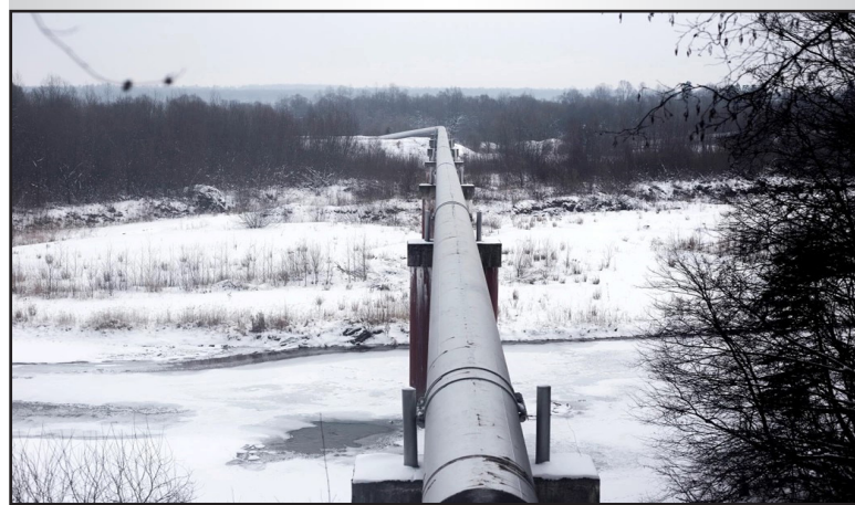
A section of the Soyuz gas pipeline near Ivano-Frankivsk, Ukraine, in 2014.
